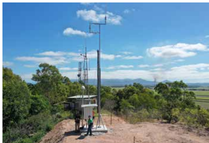
New GPS Basestation installed at Warrens Hill
