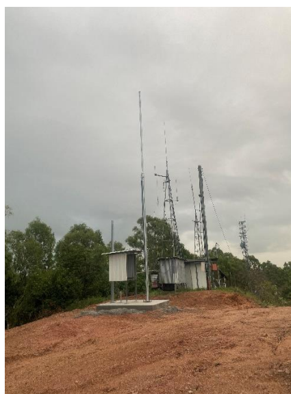
Photo above- The new HCPSL base station located at Warrens Hill adjacent to other regional infrastructure.
